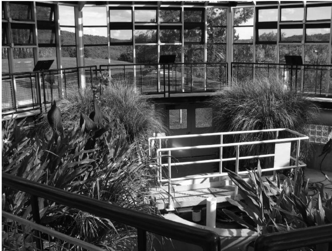
FIGURE 7.10 This artificial ecosystem, known as a Living Machine, treats toilet wastes at a rest stop on the Vermont Turnpike.
