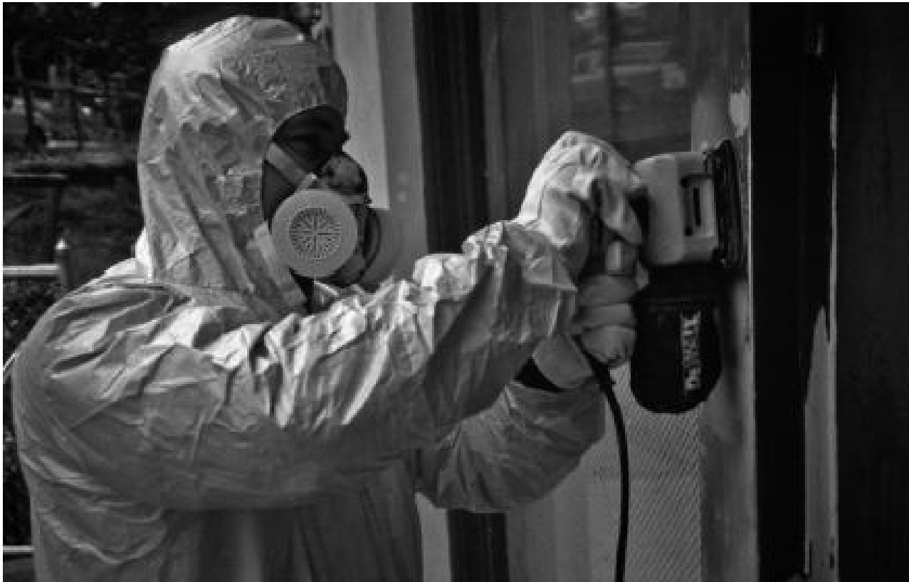
FIGURE 7.23 This worker wears protective gear as he demonstrates the use of a power sander to remove lead paint in 1999—a common renovation method at the time.
