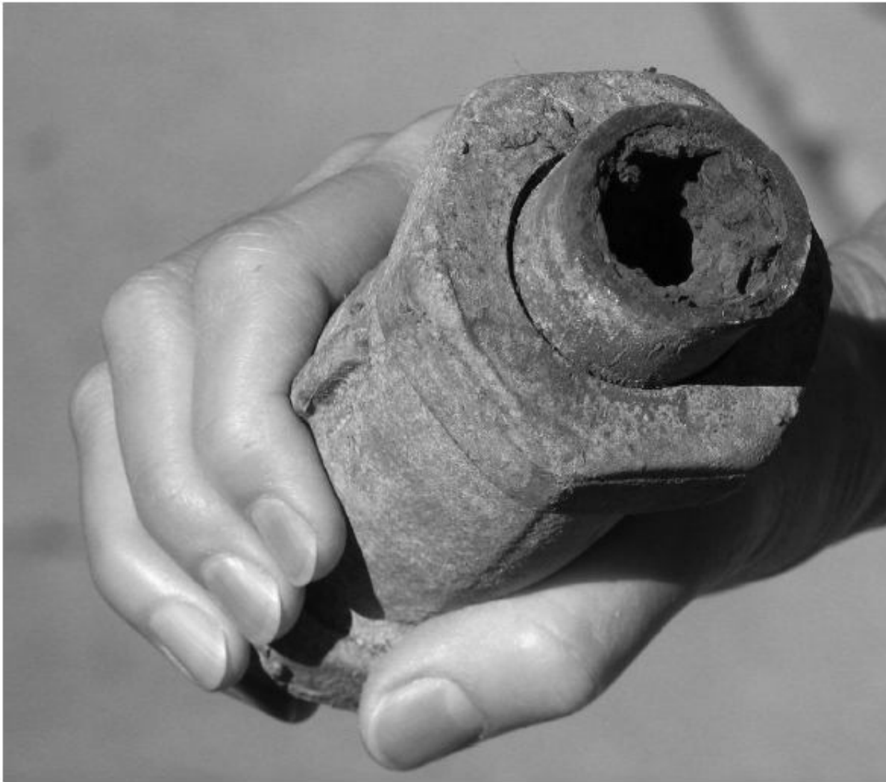
FIGURE 7.11 This 10-year-old water supply pipe has accumulated mineral deposits that make its internal surface rough.
